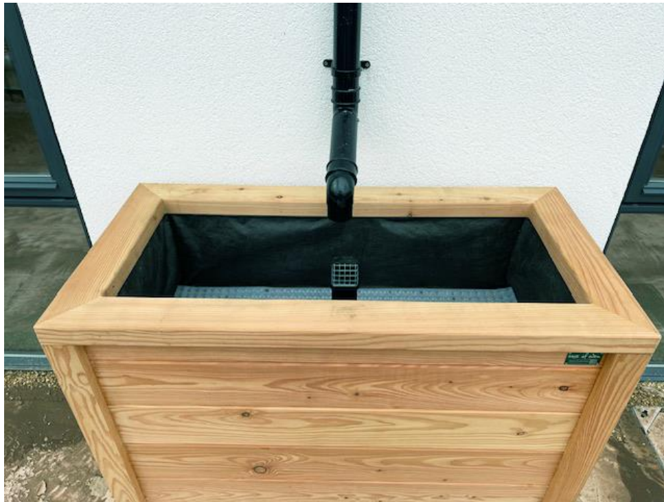
Fig 2. East of Eden Larch SuDS Rain Garden Planter with water storage area and internal drainage below a Geotextile layer
